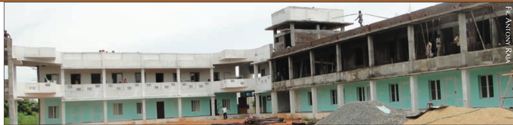
Construction continues on the Marians' new Divine Mercy Seminary in Karumathur, India. Work began in May 2010. It is expected to be finished in 2013 and will house 40-45 students, five to seven priests, plus staff.
